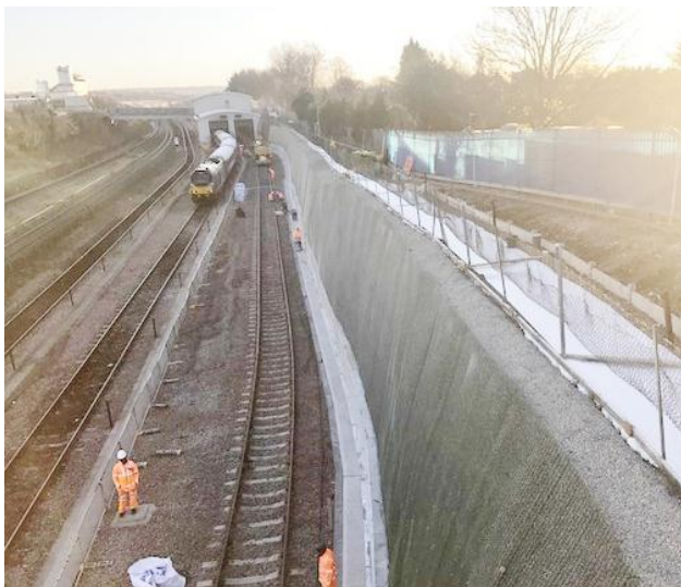
Finished retaining structure. The system using Deckdrain gained Network Rail engineer approval after trial
